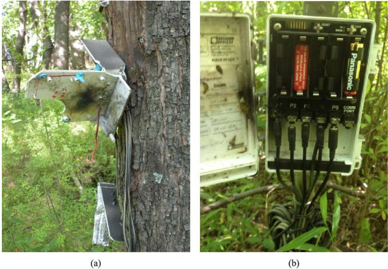
Figure 86. (a) Remnants of node 2115 enclosure. (b) EM50 data logger with damage to port 1 (P1) and scorching to enclosure door.
