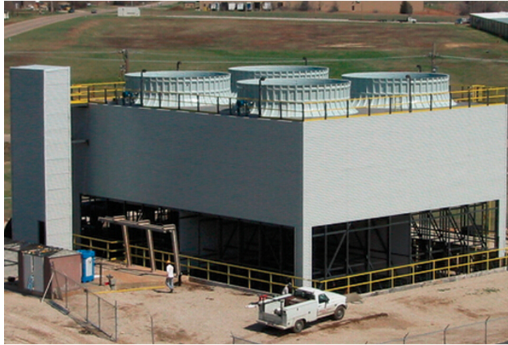
Figure 1.3 Cooling tower with pGFRP structure (Midwest Cooling Towers 2015)
