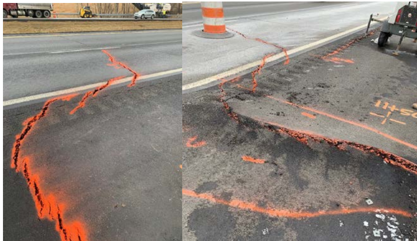
Figure 77 Image of tensile crack that formed at EB 11+05 on February 5 (left) and compression bump that formed in shoulder at EB 11+05 on February 6 (right)
