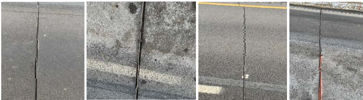
Figure 81 Field images of open pavement joints during undermining
