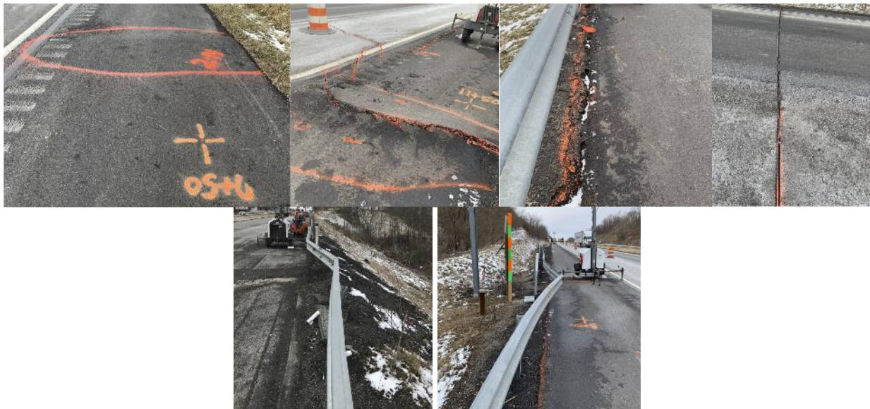
Figure 51 Field images of observed features on February 14 th from left to right; westbound blow-up, eastbound blow-up 7-inches tall, eastbound separation of pavement from soil, joint width of 0.75-inches, sheared guiderail in westbound lanes, sheared guiderail in eastbound lanes
