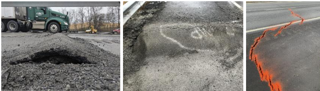
Figure 49 Field images of observed features on February 5 th from left to right; eastbound compression bump/blow-up 1-foot tall, westbound blow-up, and eastbound transverse crack 2.5-inches wide
