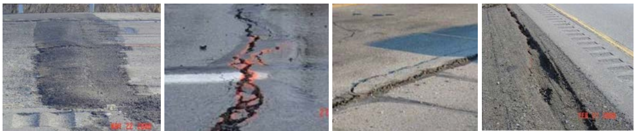
Figure 22 Examples of surface damage on I-79 caused by Emerald and Cumberland undermining showing a) compression bump, b) transverse crack, c) joint faulting, and d) lane-to-shoulder separation (Iannacchione et al., 2008)
