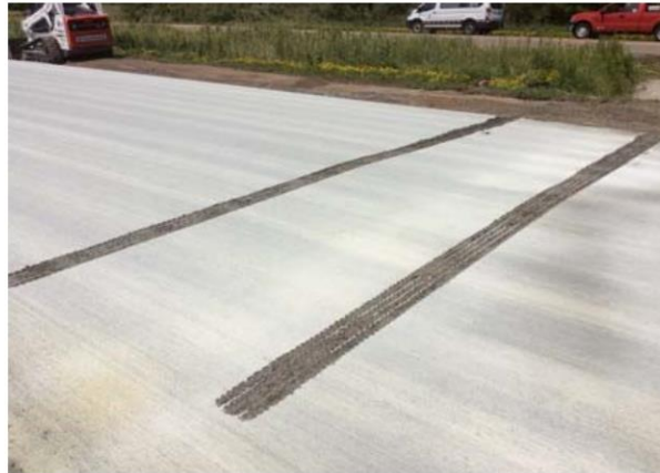
Figure 13: Damage in Cell 624 due to early loading
