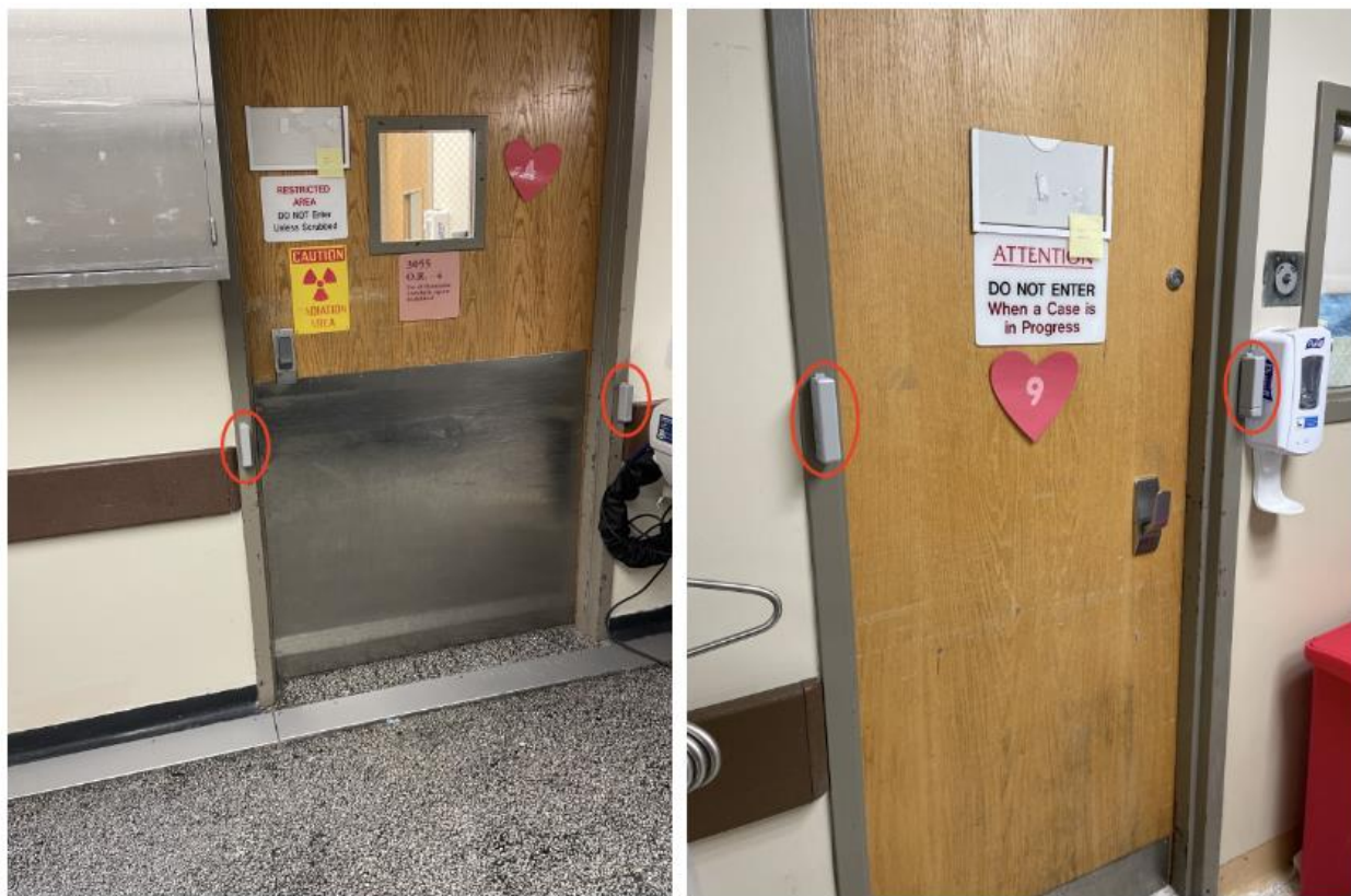
Figure 3: Device Placement on Doors of ORs 4 and 9
