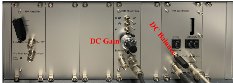
Figure 37: Wavetrain Control Box DC Knobs
