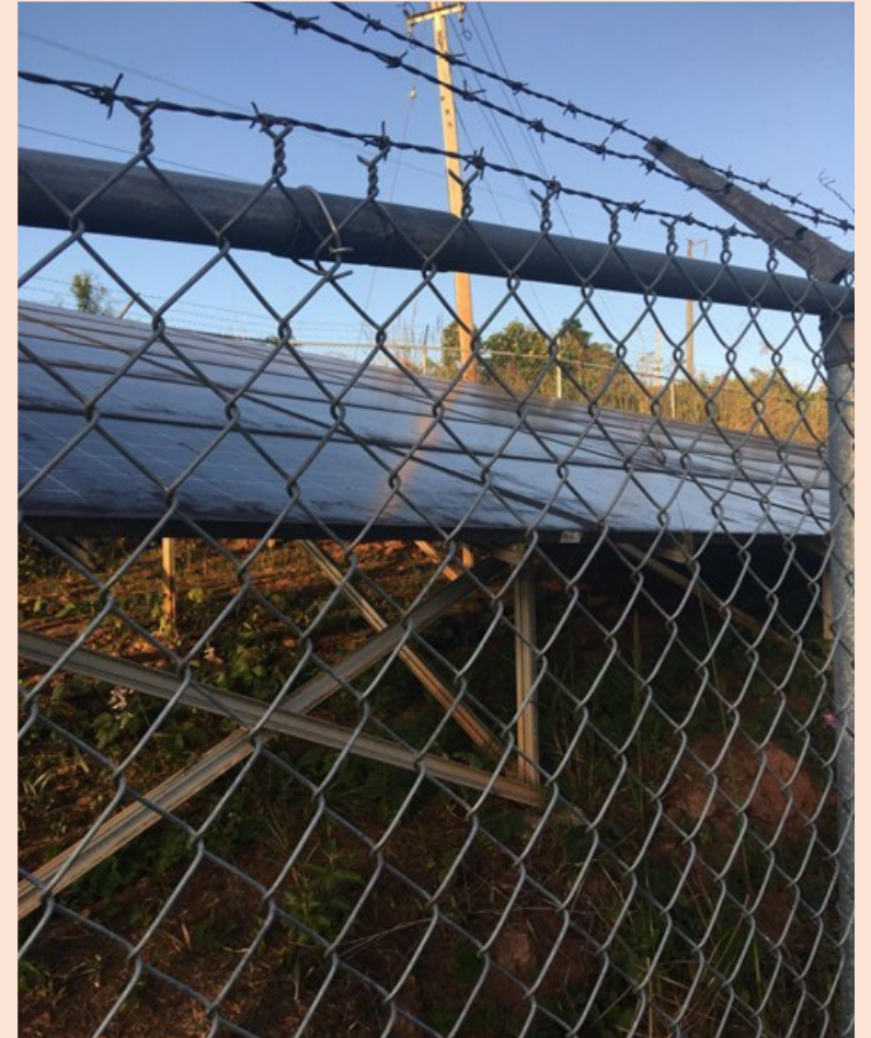
Solar panels installed for the Community Water System in Corcovada, Puerto Rico. Image credit: Research Team photo, 2020.
