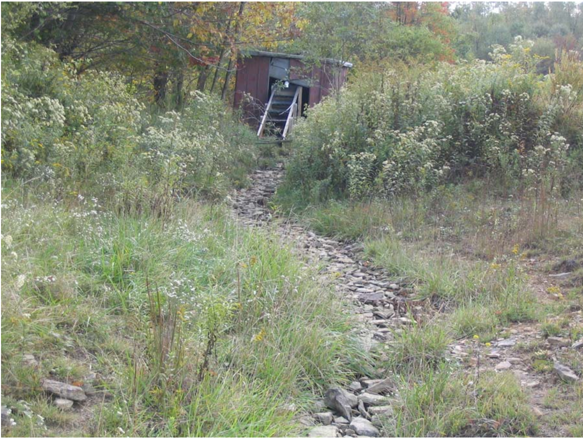
Figure 21. The caustic soda mixes into the water as it tumbles down the steps in the structure in the background and as it flows over the large rocks on its way to the first settling pond.
