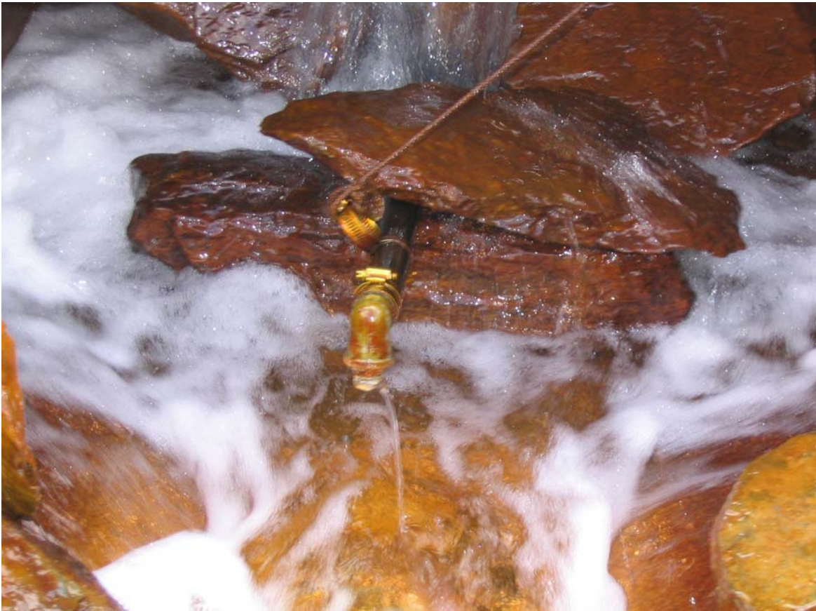
Figure 20. The caustic soda is gravity feed into the mixing box and controlled by a manual valve
