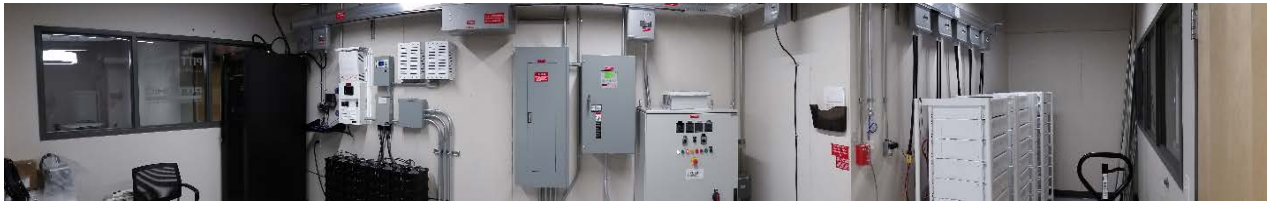
Figure 8. Electrical Equipment within the Pitt Ohio Harmar Facility
