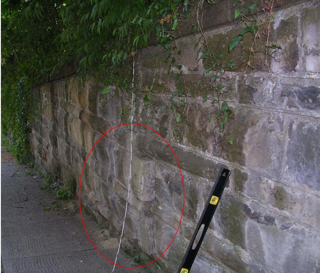
Figure 15. A "popout" failure in a gravity wall in Edgeworth, Pennsylvania. (Photo property of J. Boward)
