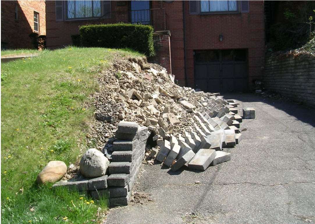
Figure 17. An overturning/toppling failure in a dry-stacked modular block wall. (Photo property of J. Boward)
