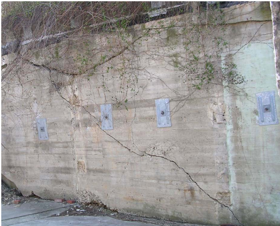
Figure 12. Tiebacks used to strengthen a failing retaining wall in Pittsburgh, Pennsylvania. (Photo property of J. Boward)
