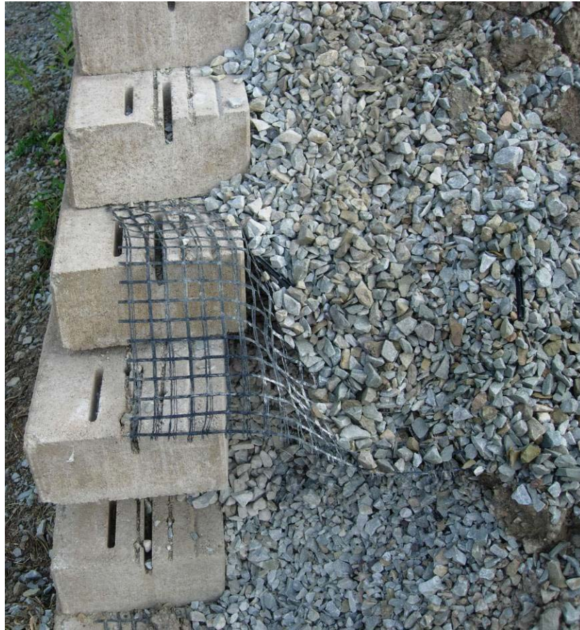
Figure 10. Settlement may induce failures in mechanically stabilized earth walls. (Photo property of J. Boward)
